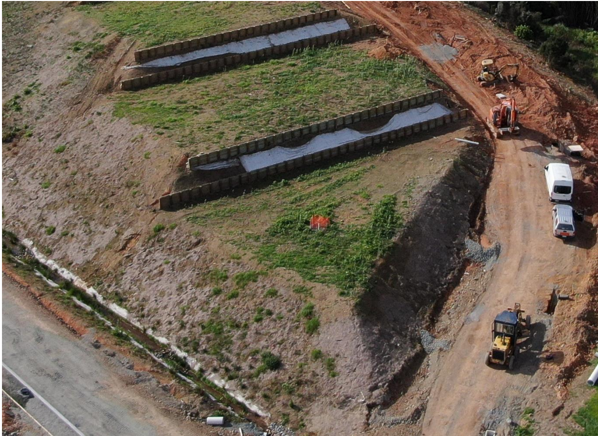
Figure 5 - Lot 1 and Lot 2 during the construction phase . Note the location of the retaining walls and batters on the left and right hand sides (west and east). Source CES Ltd.
